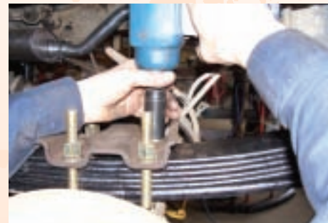
The rear leaf spring retention brackets are bolted on using the new hardware that comes with the kit. It is important to be sure and check that these bolts are still tight after the first 500 miles of driving on the new suspension.
