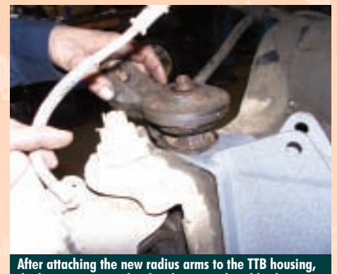
After attaching the new radius arms to the TTB housing, the lower anti-sway bar brackets are placed back into position followed by the lower coil seats.
