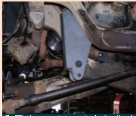
The TTB axle now rests in its new pivot brackets. Note the 6" lift hole also in this pivot bracket.
